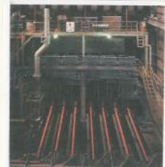
Contnuous casting plant
