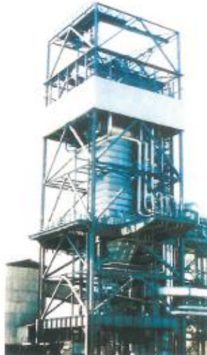
Direct reduction plant
