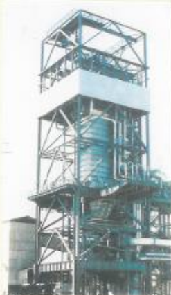
Direct reduction plant
